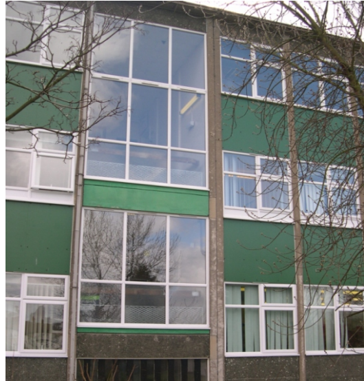
Typical stairwell at a school, note the balustrade / barrier on the internal face
